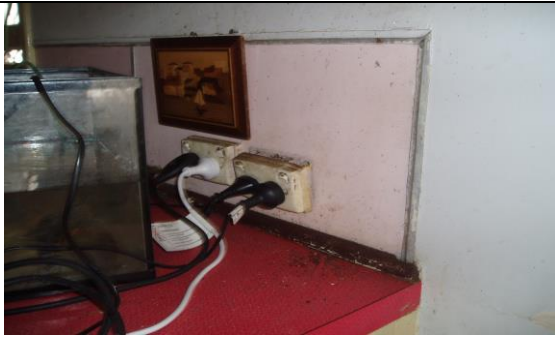
Powerpoints coming off the walls in many rooms in the house.
