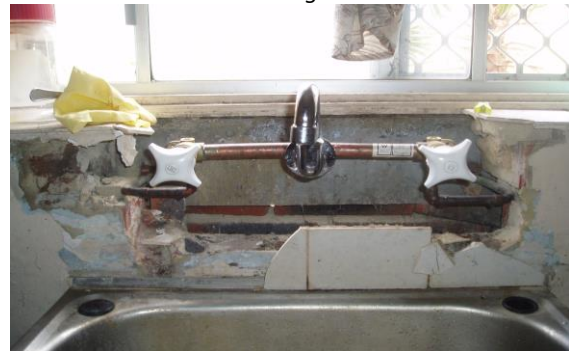
Laundry sink with exposed blue asbestos fibres
