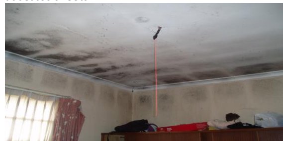
The ceiling is leaking and had not been repaired and is thick with mildew and also no light fitting.
